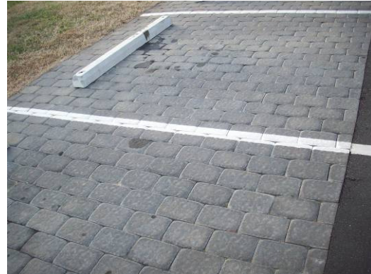
Permeable pavers are installed in the parking lot of Willow Ridge Apartments in Morganton. Stormwater carrying pollutants will infiltrate through the pavers rather than washing off into nearby waterways.
