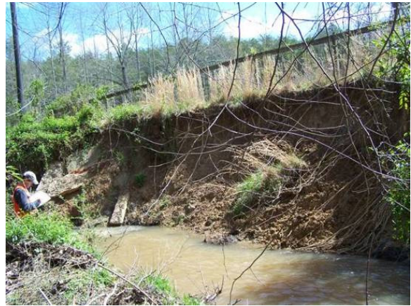
Erosion site along Hunting Creek.
