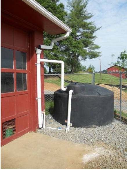
An above ground cistern located at the City of Morganton Parks and Recreation maintenance building catches runoff from the roof. The high pressure water is used to clean equipment.
