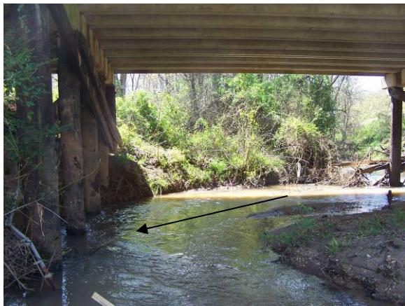
Bridge crossing not aligned with flow of stream (As indicated by arrow) causing stream bank erosion.
