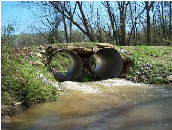
Structural crossing with double culverts creating a barrier to fish migration.
