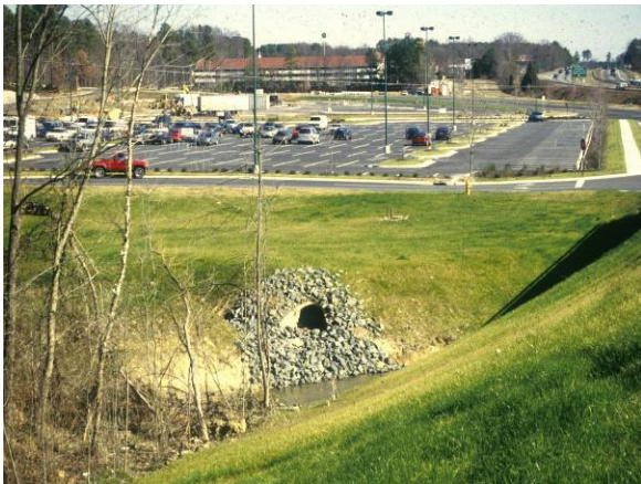
Stormwater running off parking lots is directed to the stream channel through a series of storm drains, underground pipes, and outfalls.
