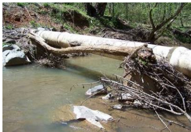
Pipe utility crossing Hunting Creek above stream with debris pile behind pipe. Also note erosion along stream bank
