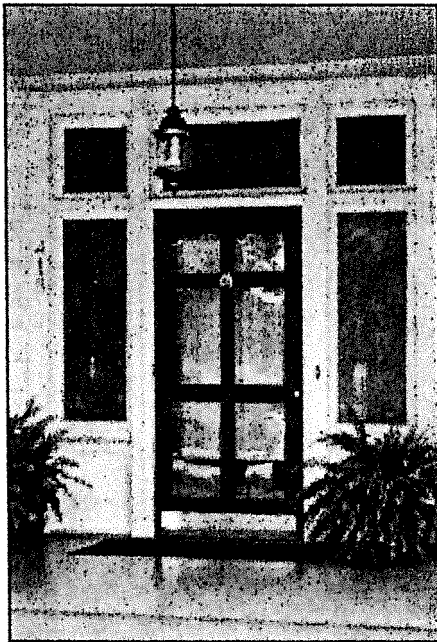
Above, a wooden storm door with glazed panels increases the energy efficiency of this front entrance. In the photo on the left, operable shutters, storm windows, and wooden interior blinds all illustrate appropriate energy-conserving options for an original wooden two-over-two window sash.
