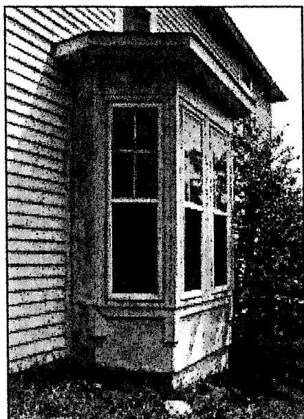
The vertical proportion and pane configuration of these original wooden windows (now protected by storm windows) reinforce the proportion and character of this side bay.
